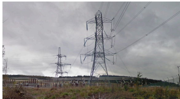
Blackhillock substation view from the land entrance
